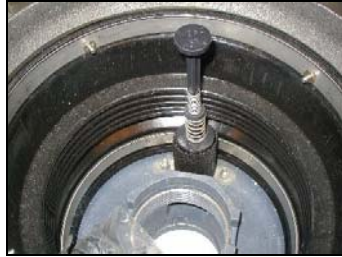
Spill bucket drain valve
