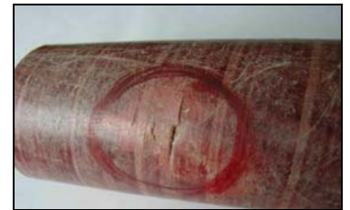
Fiberglass piping is cracked
