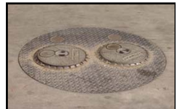
Fill and vapor recovery lids installed within a larger sump lid
