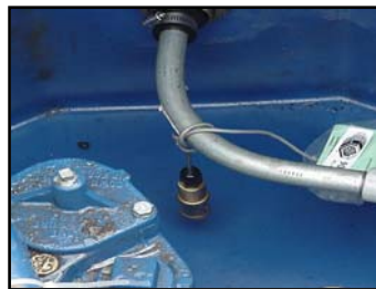
Liquid sump sensor
