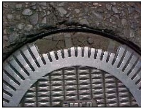
Cracked spill bucket lid
