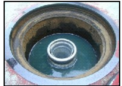
Spill bucket that contains liquid
